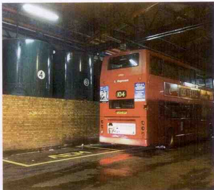
Latest Envirox dosing system installed in London depots.
